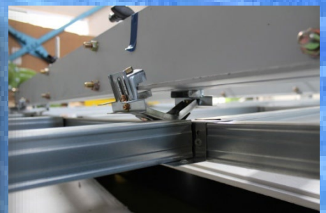
Destruction of ceiling
