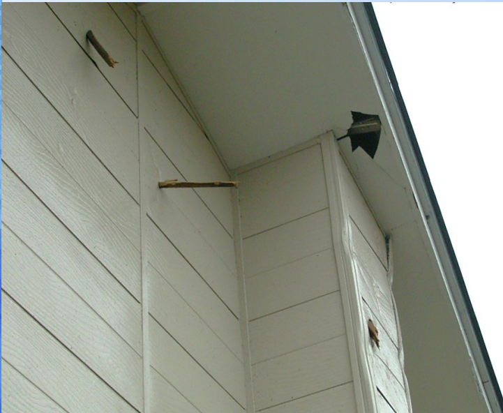
Tornado-borne flying debris penetrating exterior walls (Atsuga, Hokkaido, 2004)
