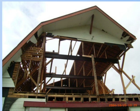
Tornado Damage, Monbetsu, Hokkaido, 2004
