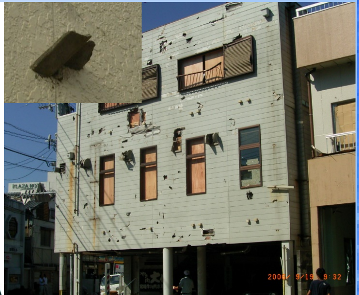
Collision marks caused by tornado-borne flying debris impacting walls (Nobeoka, Miyazaki, 2006)
