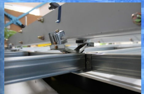
Destruction of ceiling
