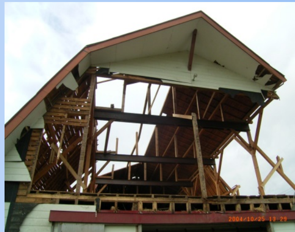
Tornado Damage, Monbetsu, Hokkaido, 2004
